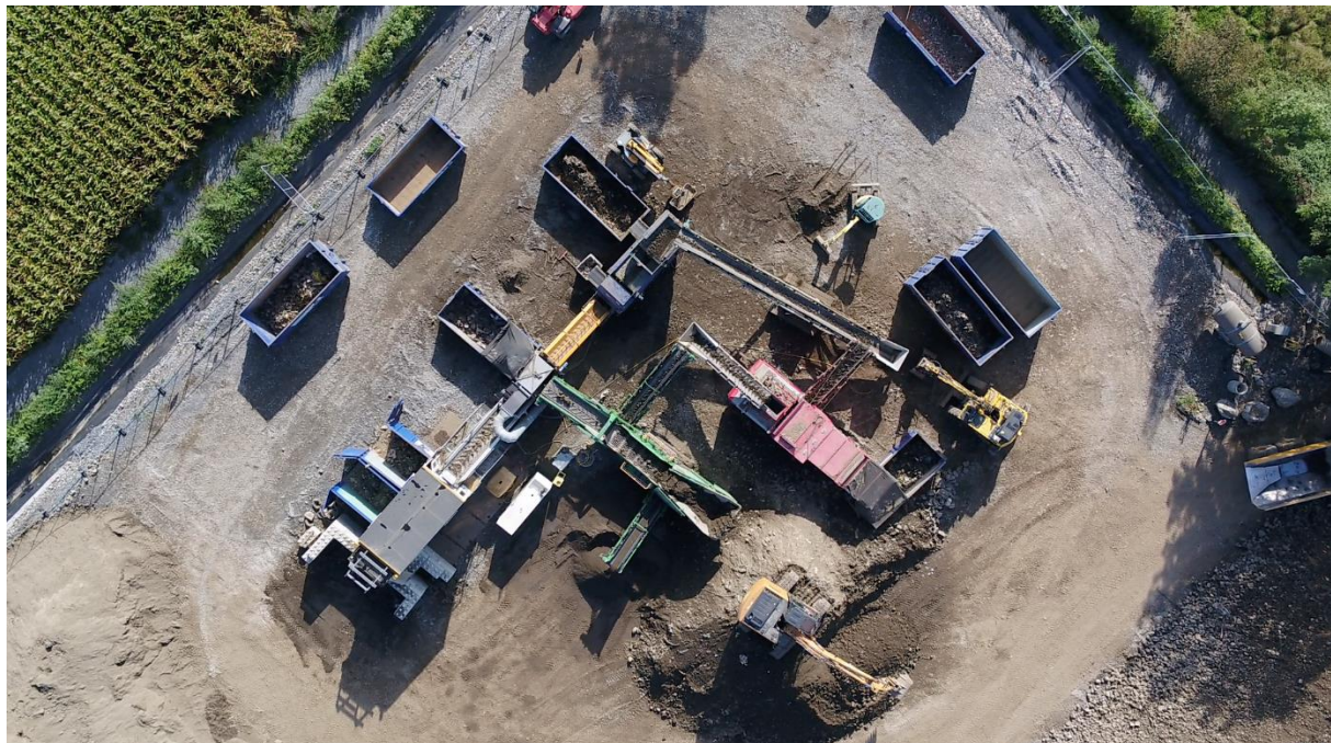
Figure 12-8 UAV view of the sorting platform (Credit photo: Conseil Départemental des Pyrénées-Atlantiques).
