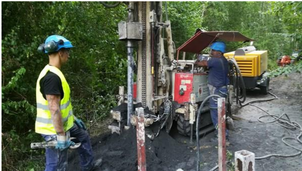
Figure 5-1 Down-the-hole hammer drilling in the fly ash deposits of the Onoz industrial landfill, one of the RAWFILL pilot site (Credit Photo: Atrasol).
