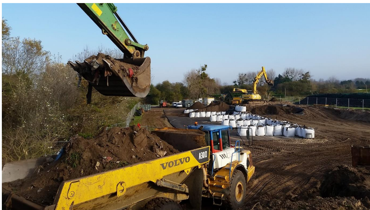
Figure 12-5 Landfill mining operations on la Samaritaine landfill. On the back, the sorting platform which is located next to the site. The asphalted area was used to store the fine fractions while waiting for the results of the geochemical analyses.
