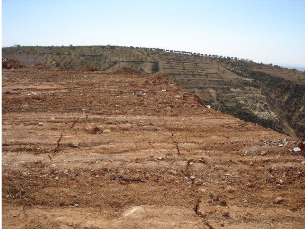
Figure 8-2 Horizontal cracks at the top of a landfill attesting stability problem (Credit Photo: Atrasol).
